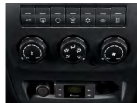
Control panel for air conditioning and heating
